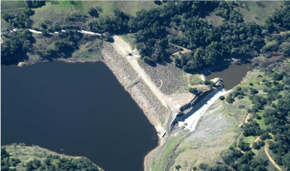
Coyote Dam and Reservoir, currently the second largest by volume operated by SCVWD, is located on the Calaveras Fault.
